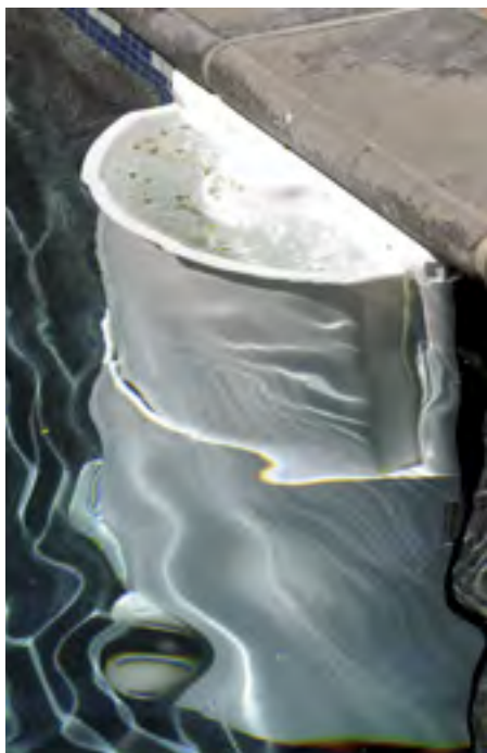
The retrofitted Ecoskim self-levelling pool skimmer
