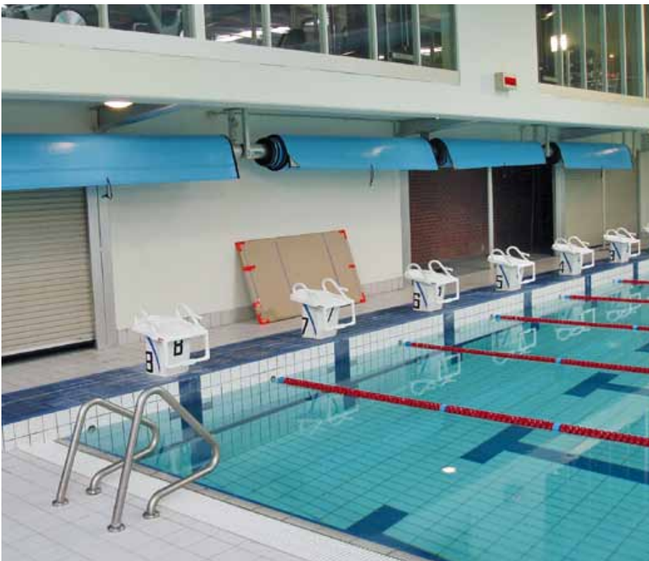
The covers had to be built inline because of the limited space
